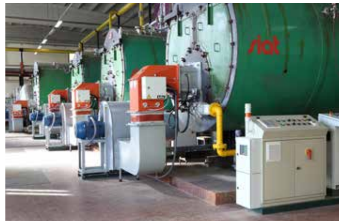
HOSPITAL HEATING Burner models: No. 2 IB 650 G ME CO V, No. 2 IB 1200 G ME CO V - electronic modulation - inverter and CO control NO x <100mg/kWh
